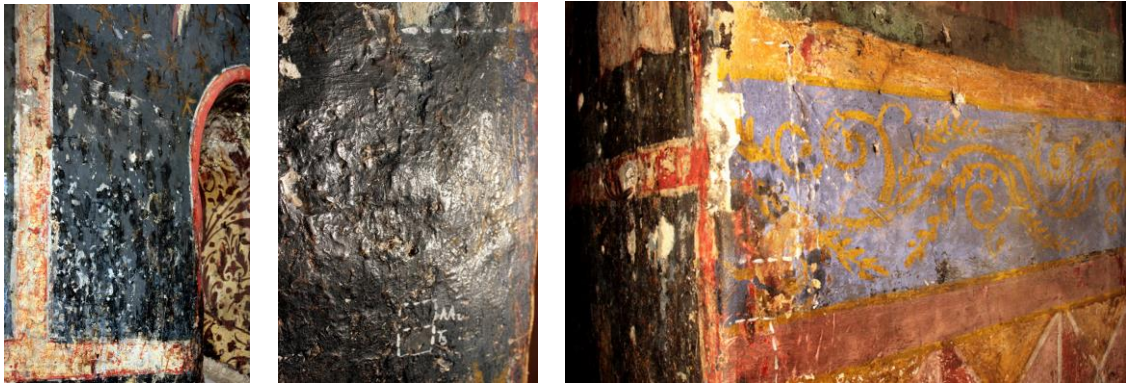
Figure 17. The “raindrops” wax deposits on the north wall Figures 18, 19. Stratified and polished wax deposits; Repainting using protein-based paint in the area of the ornamental belt
