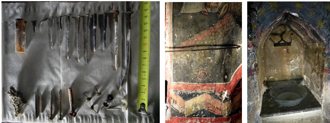
Figure 11. Foreign metallic materials taken out from the fresco Figure 12. Improved towel rack. Figure 13. The abusive “modernization” of the washing table
