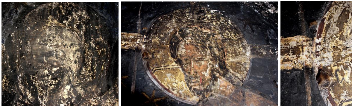
Figure 23. The loss of adhesion of the pigment of the paint payer, before the restoration Figures 24, 25. Flaking and pulverization of pigments, after the first cleaning intervention
