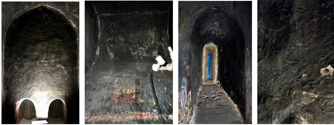
Figures 7, 8, 9. Opaque layers of superficial deposits on the scene “Christ in the tomb”, on the inner face of the vaulting, also in the window on the north wall. Figure 10. Spider webs - detail
